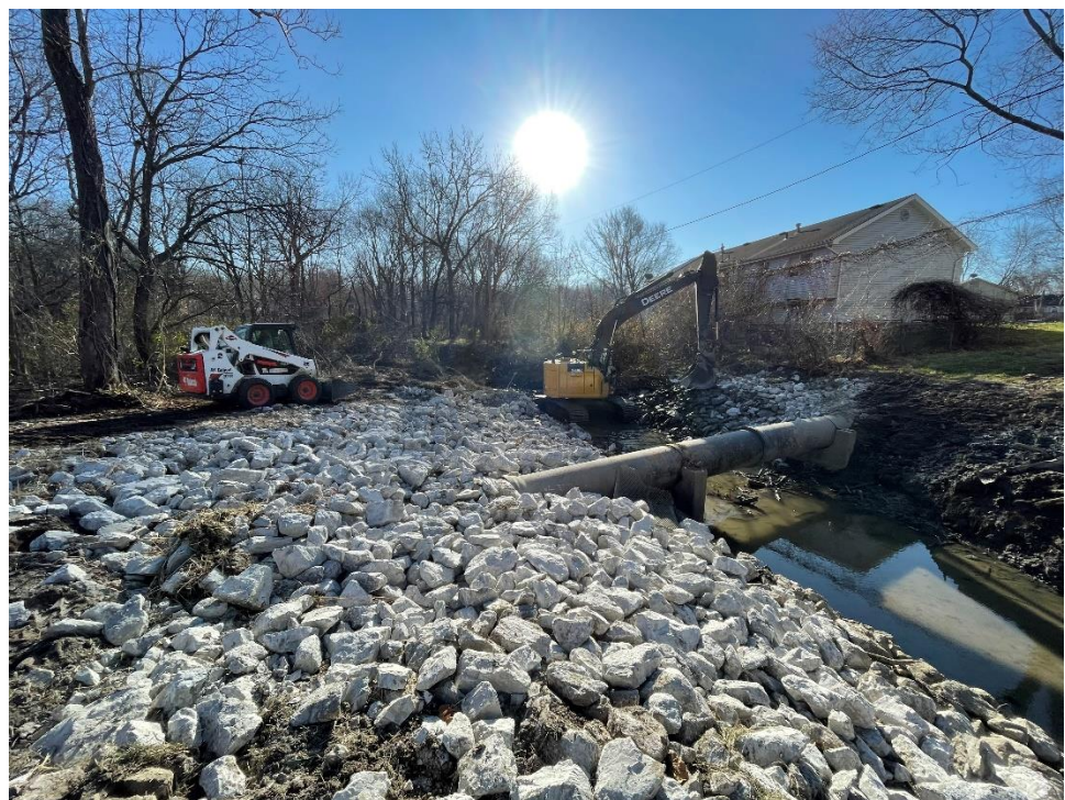
PCRSD staff stabilized the Walnut Creek bank along the sewer line aerial crossing. The bank was scoured and risked undermining the line and upstream manhole.
