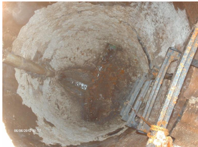
Figure 3: A manhole with severe corrosion discovered during the SSES. It was rehabilitated in 2014.
