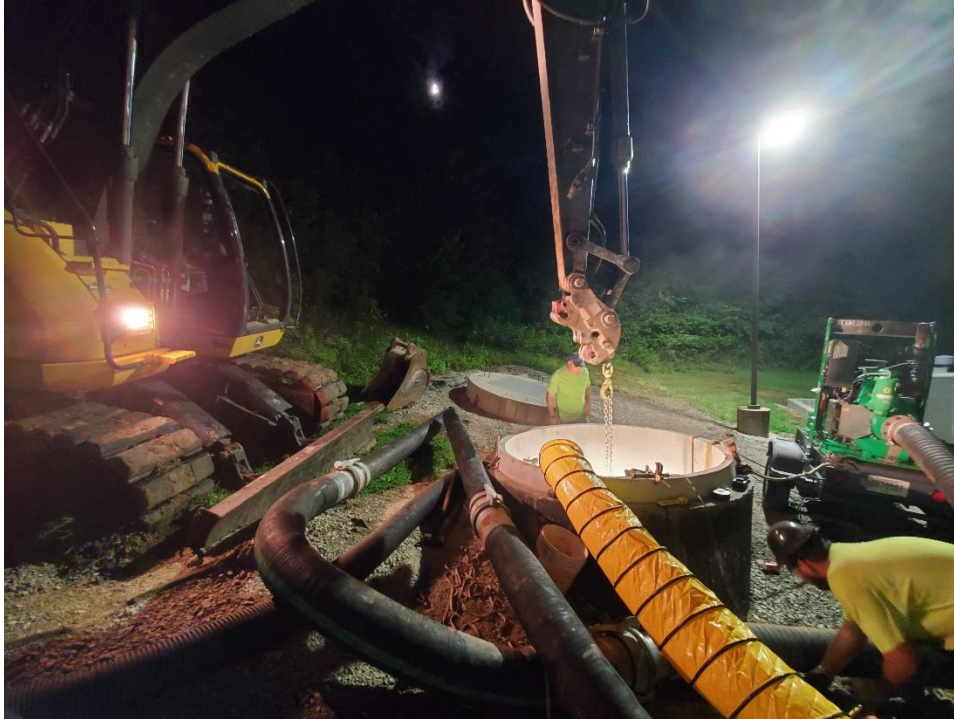
She Digs It employees prepare the flow meter pit at the Brush Creek WWTF for bypass pumping while the headworks channel was rehabilitated and lined with epoxy coating.
